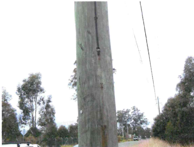
Copper thieves cutting and taking earths from power poles means there is inadequate connection to the earth placing persons and the electricity network at risk. This example occurred in Prospect NSW part of Endeavour Energy's franchise / network area. Crime Stoppers is urging anyone with information about copper theft in their area to report it anonymously to Crime Stoppers on 1800 333 000.
