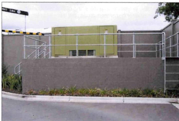
Figure 51 - Example substation raised above 1:100 flood level
